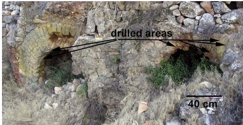
Fig. 3. Photograph of kiln Bu at La Buada with indication of the drilled areas below the arches that supported the grid.
